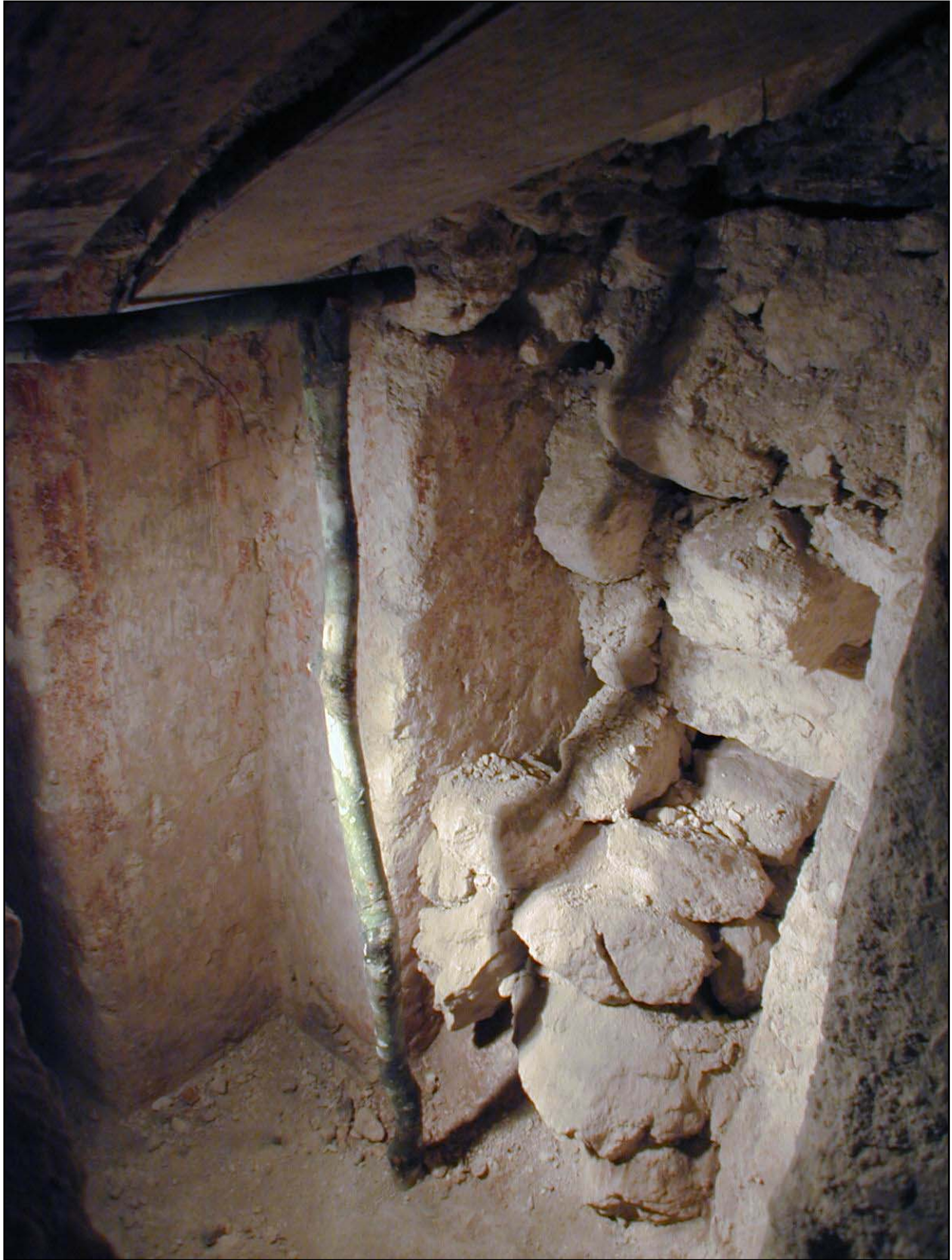
Figure 10 Rubble-filled doorway to Structure 1 room 3
